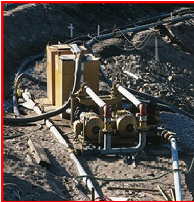
Plate 2.7 Pump used in Eductor well point system
